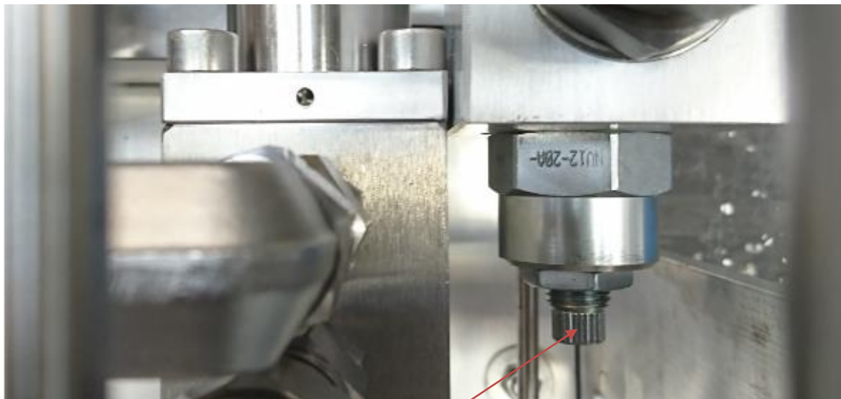
Hydraulic flow control valve
